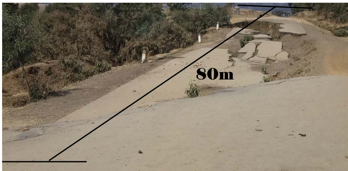
Figure 3.4: slope failure/slide characterize
