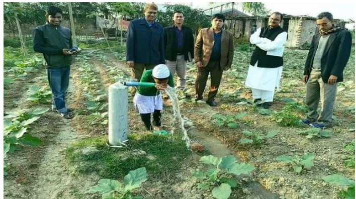
Fig. A faucet with underground uPVC irrigation pipe line in dug well scheme.
